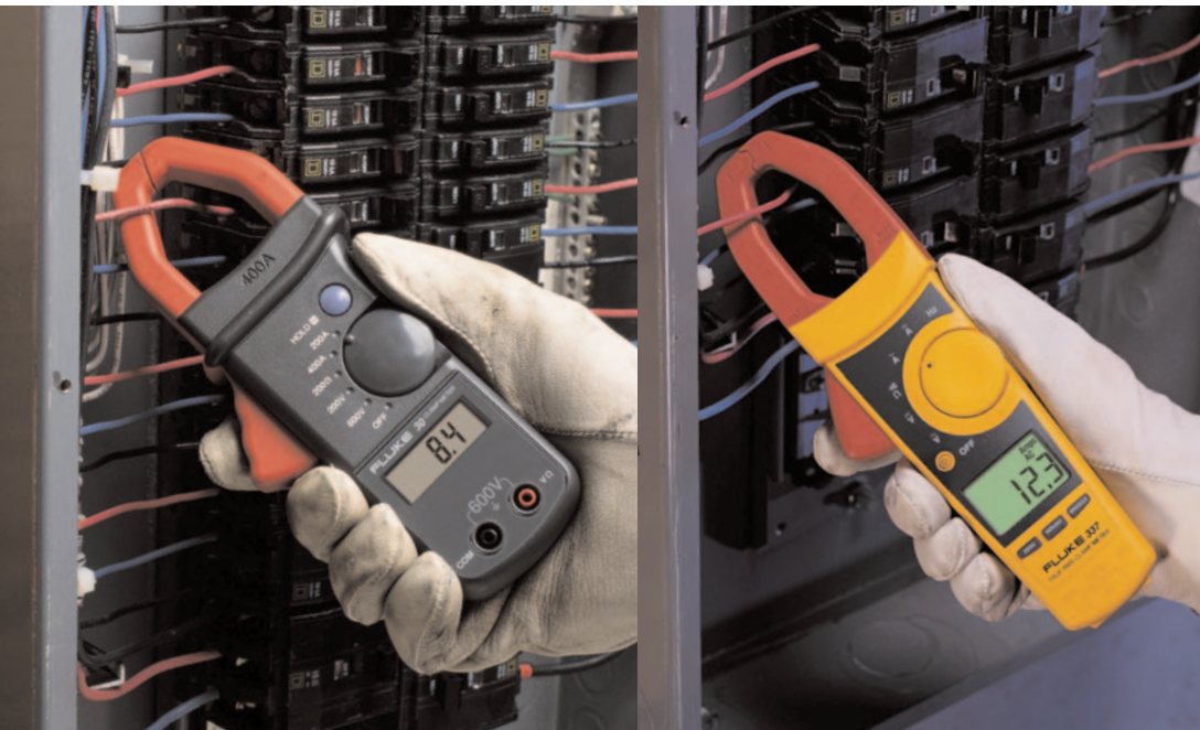
Figure 1. One current—two readings. Which do you trust? The branch circuit above feeds a non-linear load with distorted current. The true-rms clamp on the right reads correctly but the average responding clamp reads low by 32 percent.
