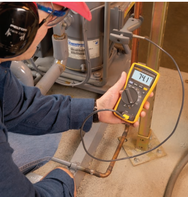
Checking hot refrigerant gas temperature going up to the condenser with a pipe clamp and a DMM.
