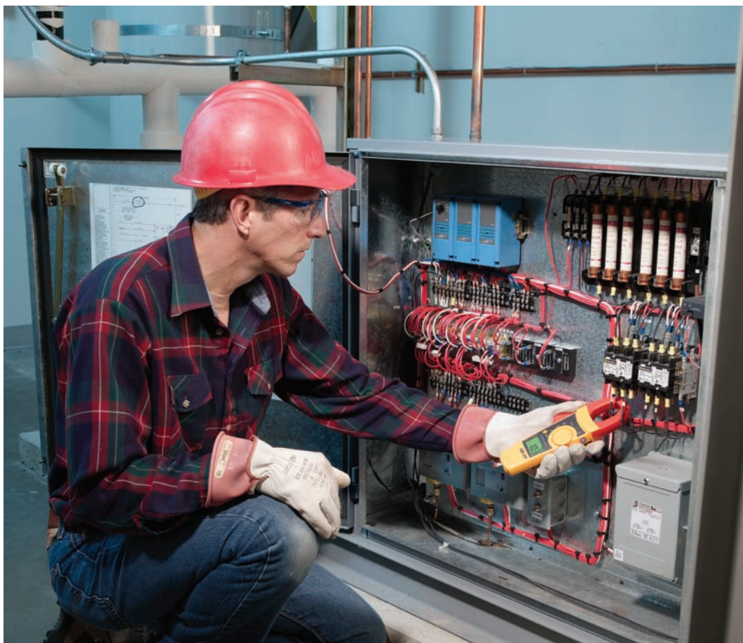
Checking running current on the compressor controls.
