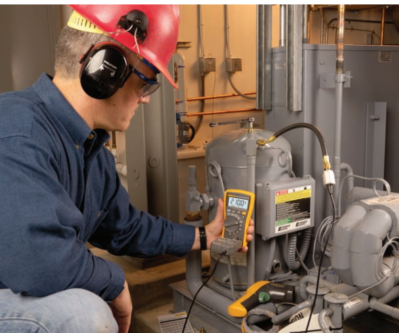
Using a multimeter and a pressure module to check head pressure.
