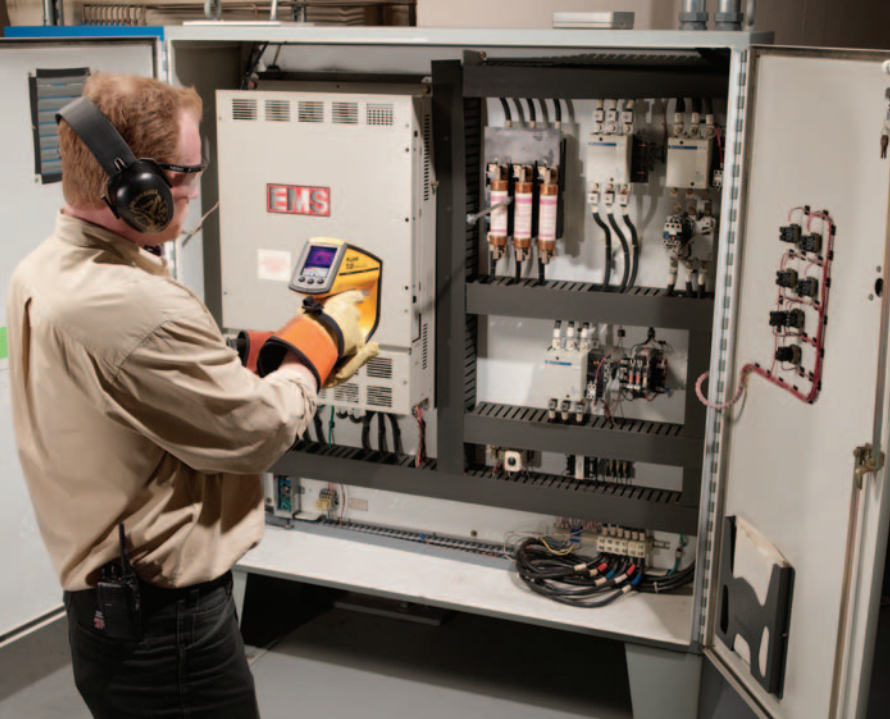
Kevin Halligan uses the Fluke Ti30 Thermal Imager to quickly check for hotspots on key equipment.
