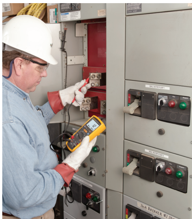
Steve Uhrich tests resistance of drive cabling.
