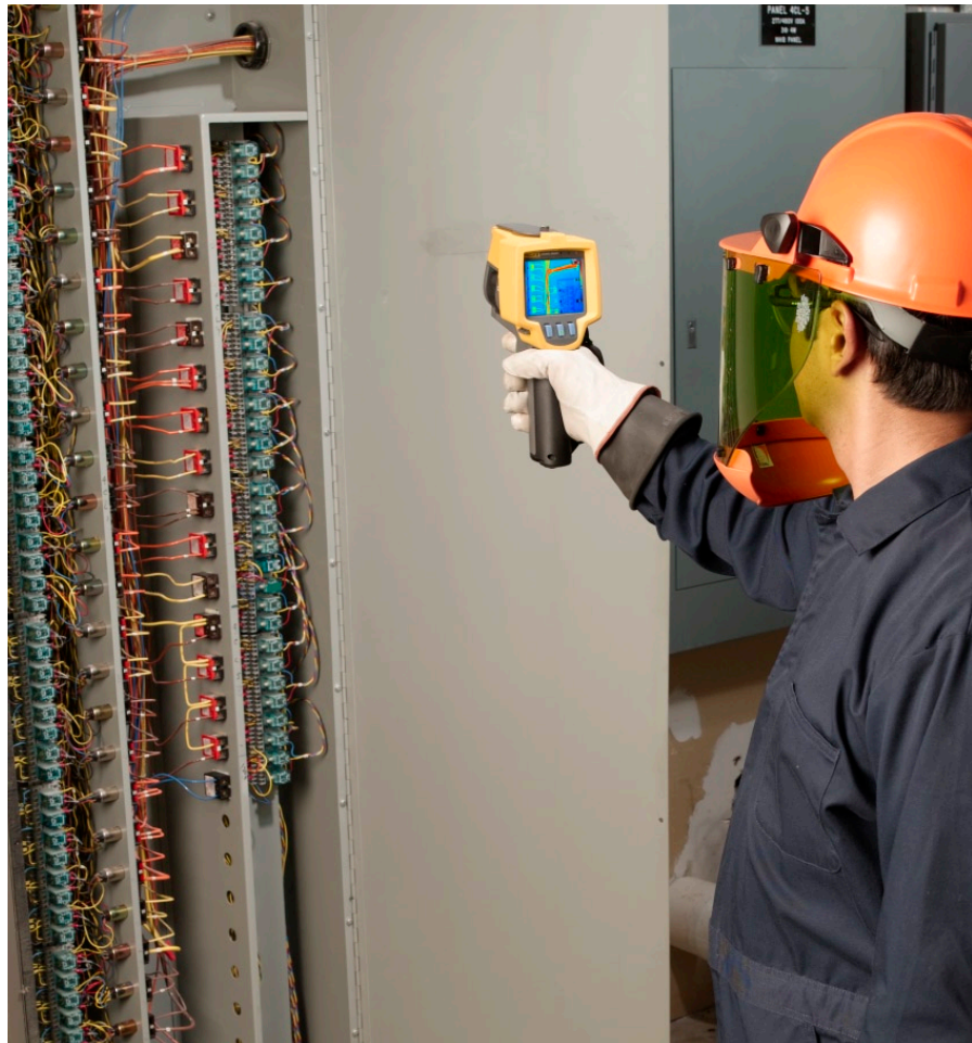
Use thermal imagers to check energized components for hot, loose or corroded connections.
