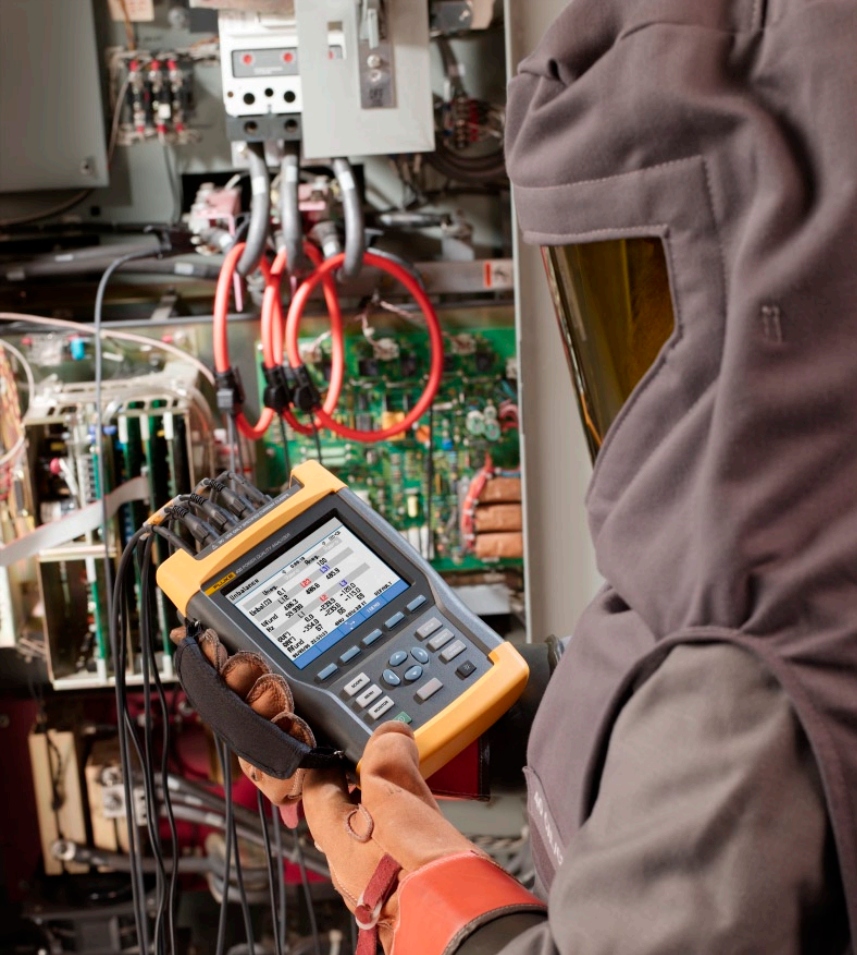
Periodically examine power quality for voltage sags, harmonics and other causes of overheating.
