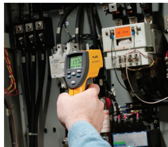
Circuit breakers – check for hot spots before they trip.
