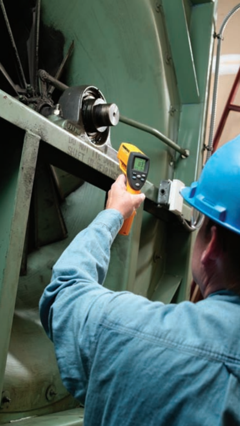
Motors: Unusual heat readings on a bearing assembly can indicate wear or inadequate lubrication. Investigate further!
