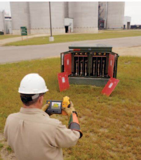
Bringing thermography in-house allows Weyh to help protect expensive equipment by scanning the ACEC-owned facilities on the sites of key co-op members.
