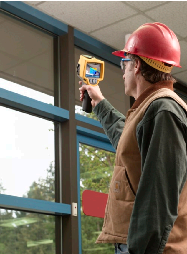
Checking for moisture within the wall surface with a Fluke InSight Thermal Imager.
