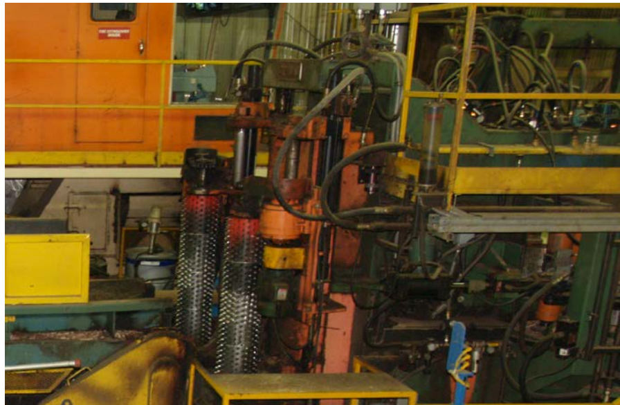
Preventive maintenance applications for Fluke thermal imaging are plentiful in an industrial environment such as this Weyerhaeuser location in Drayton Valley, Alberta.
