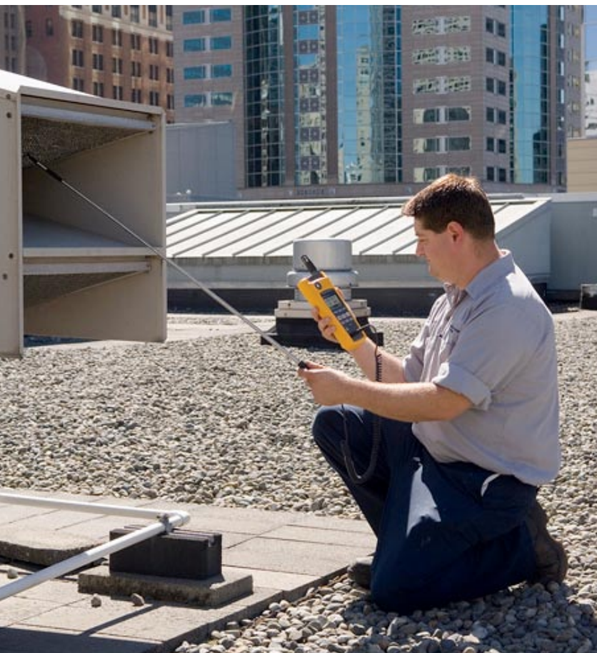
Using the velocity probe for measurements at the air intake.
