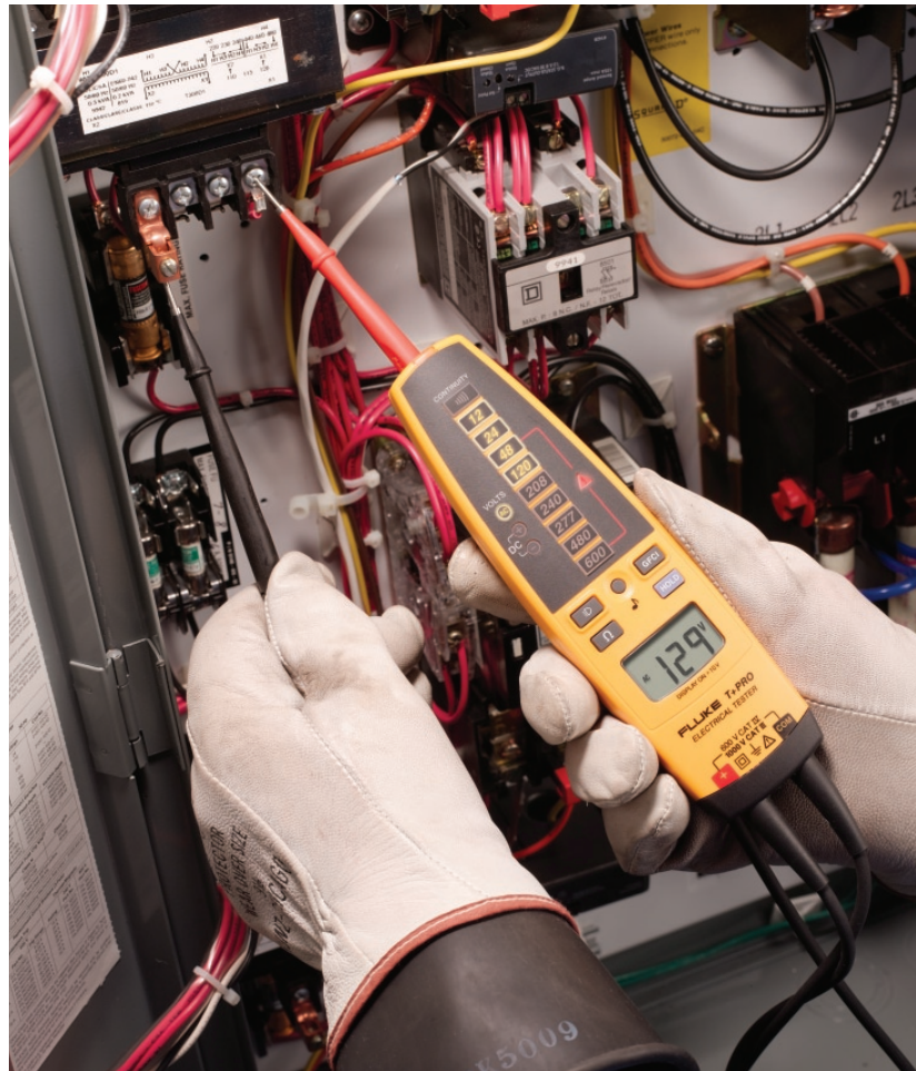
Testing control voltage on a 480 V panel controlling two small chiller pumps.
