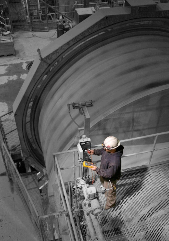
Ken Bartlett troubleshooting a flow control valve for the water addition to the Sag Mill.
