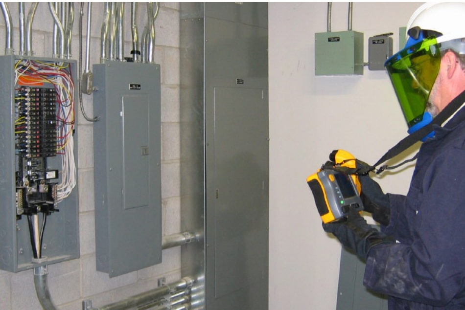
Inspection of an electrical control circuit.
