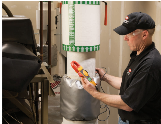
Checking temperature differences across the exchanger.
