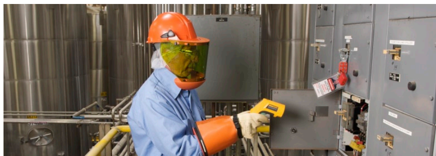
Keith Morin comparing heat signatures on MCC fuses.
