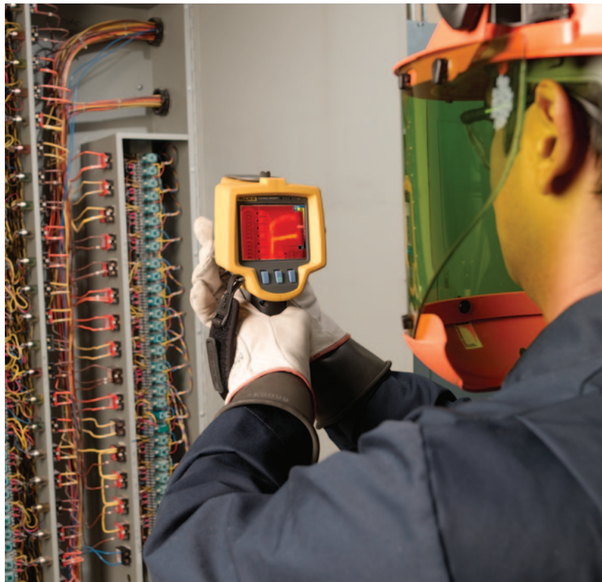
Inspection of lighting control circuits with a Fluke Ti25 Thermal Imager and appropriate PPE.
