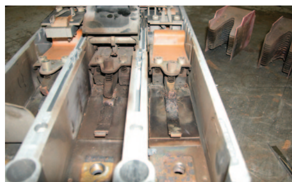
Figure 4. Molded-case circuit breaker with welded contact.
