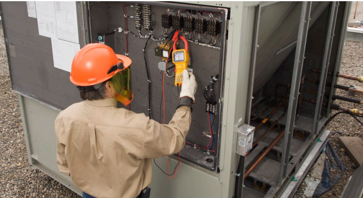
Taking a 208 V measurement on one leg of a three phase circuit for a roof-top HVAC unit.
