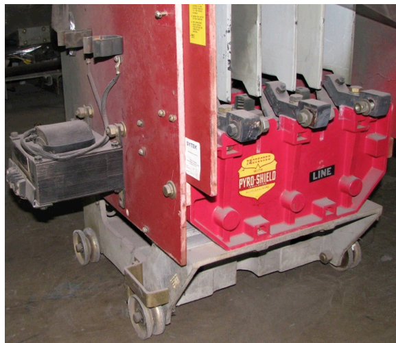
Figure 4. Note CPT Mounted on Side of 4.16 kV Starter. The 480 V Terminals Cannot Be Clearly Identified
