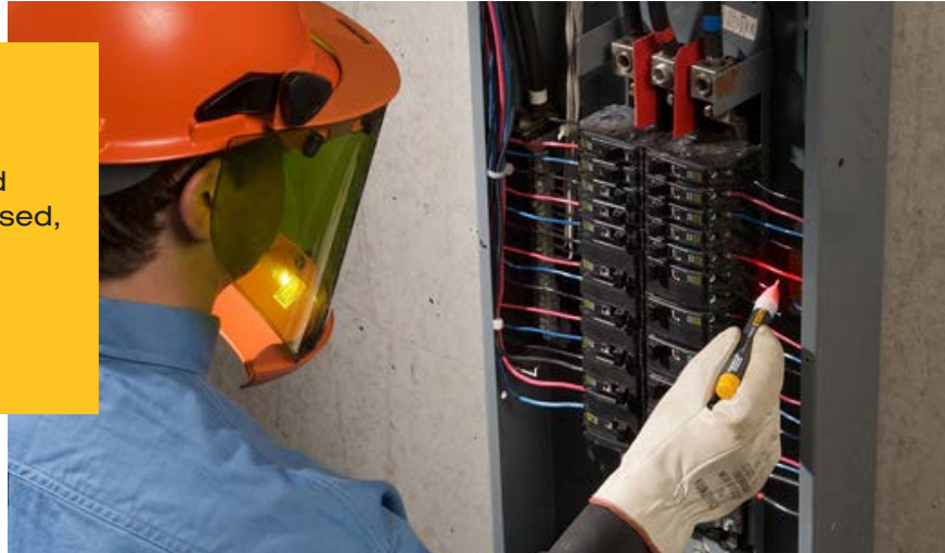
Figure 1. Use a non-contact voltage tester for your first test.
