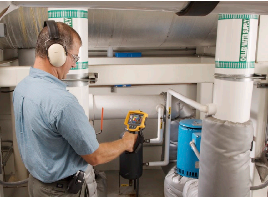
During a motor scan, Fleming noted abnormal temperatures on this unit.
