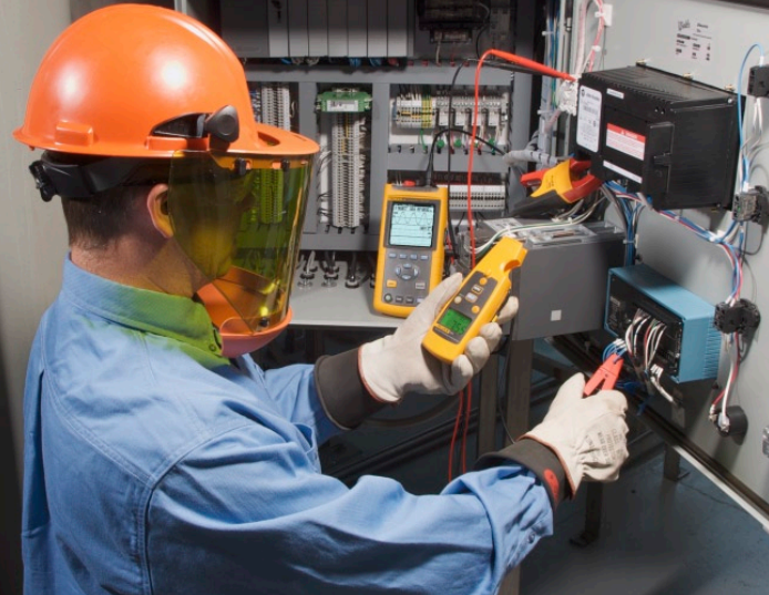
Checking conductivity meter on an A/B control box. Using the 771 mA Clamp to verify the 4–20 mA signal from the unit to chart recorder, and the using the 43B Power Quality Analyzer to check power quality into the system, looking for fluctuations.
