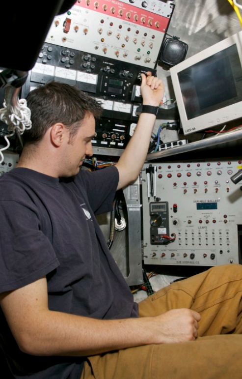
Sean Kelley switches through the various electrical systems aboard the sub, and compares the analog meters against the Fluke 77 DMM mounted in the control panel.
