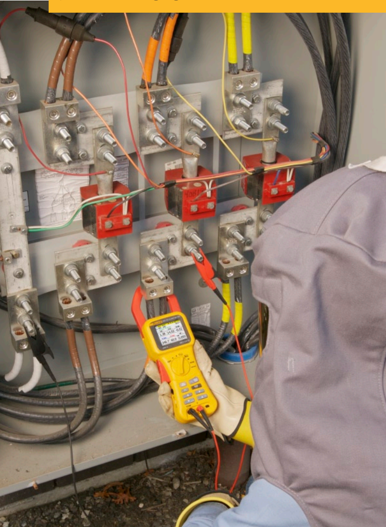
Measuring kW energy consumption will give you a more accurate bid, in far less time, than estimating off of total fixtures.
