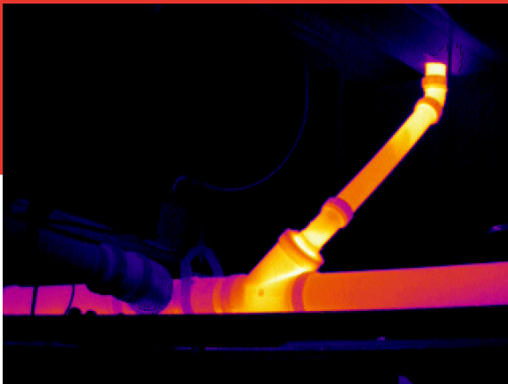
Infrared imaging shows a partial blockage in a process liquid waste drainage line. Failure to recognize a deteriorating situation could result in serious problems.
