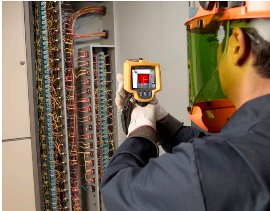
Abnormally hot electrical connections are not only an early warning of failure and a safety hazard, they’re also consuming excess energy.
