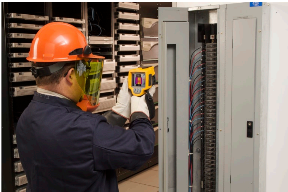
Inspecting connectors in a panel supplying video server racks.
