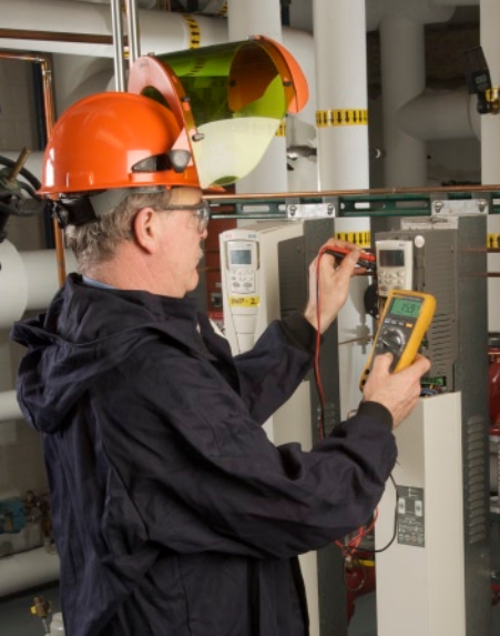
Jim Murphy, Electrical Foreman uses the Fluke 179 DMM to look at low voltage signals in the newly installed VFD for the 40+ year old steam system.
