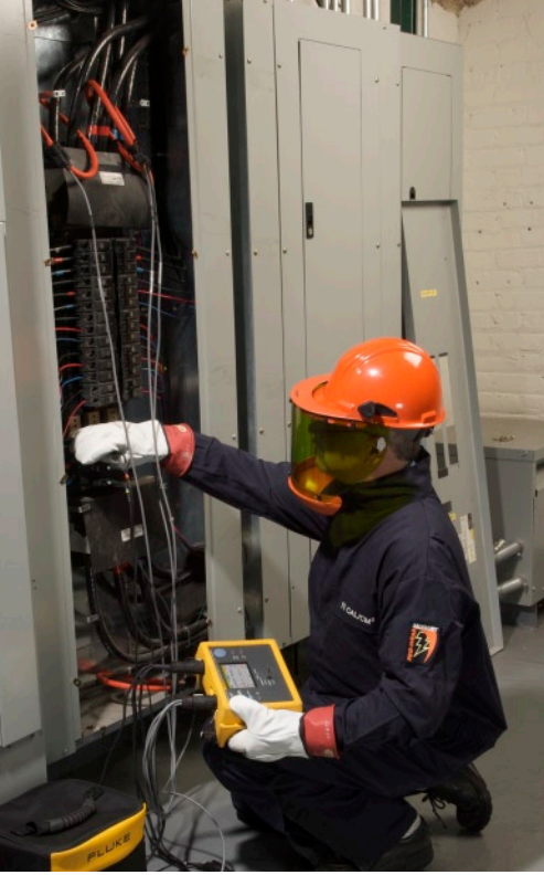
Rolf Zoeller, Electrician uses the Fluke 1735 Three-Phase Power Logger to do load studies on the hospital's electrical systems. Keeping close tabs on these systems helped the hospital achieve its ENERGY STAR rating.
