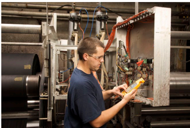
Martin uses the 773 milliamp clamp meter to check the 4 mA to 20 mA signal between an electronic temperature controller and an electric to pneumatic pressure transducer that operates a steam valve. He compares the output percentage reading on the 773 with the output that the electronic controller displays in a diagnostics mode.
