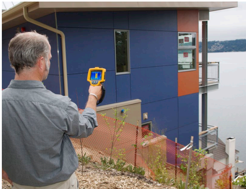
Infrared inspection of all external windows and doors can often show defects in installation or materials that contribute to energy loss.
