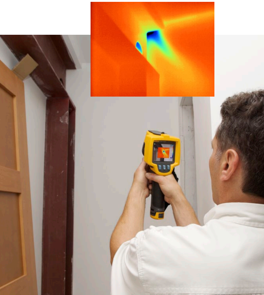
An unexpected area of air infiltration was found coming from behind a major support beam. This may have never been discovered without the use of the TiR32.
