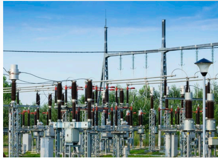
A hot spot on this porcelain terminator or pothead was easily detected with infrared. While the component itself is not extremely expensive, the cost of an outage resulting from its failure is. Here infrared not only found the problem, infrared also verified the fix.
