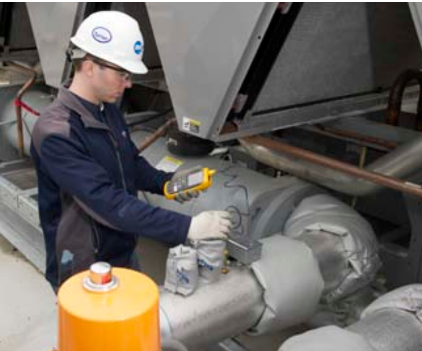
McKinstry commissioning engineer Bryan Morris checks a chiller circuit.
