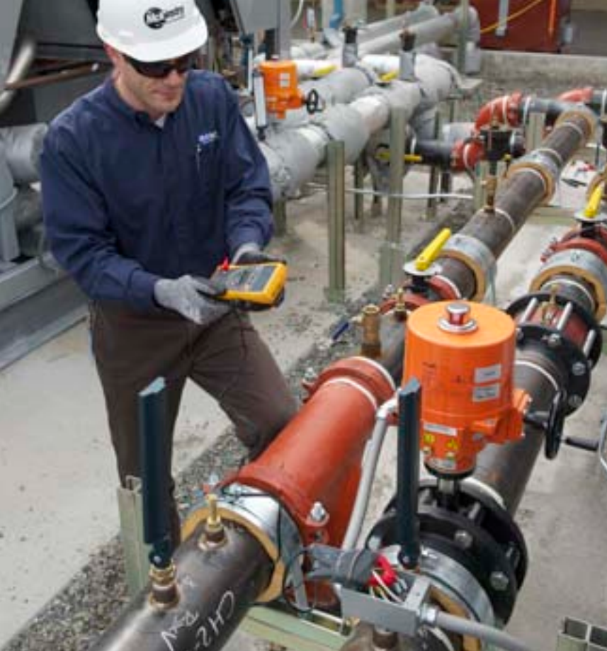
Commissioning engineer Jeff Fogel uses a multimeter and clamp accessory to verify chilled water valve operation.
