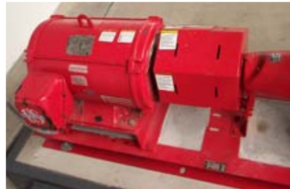
The pump is one of three components of a modern chiller plant.
