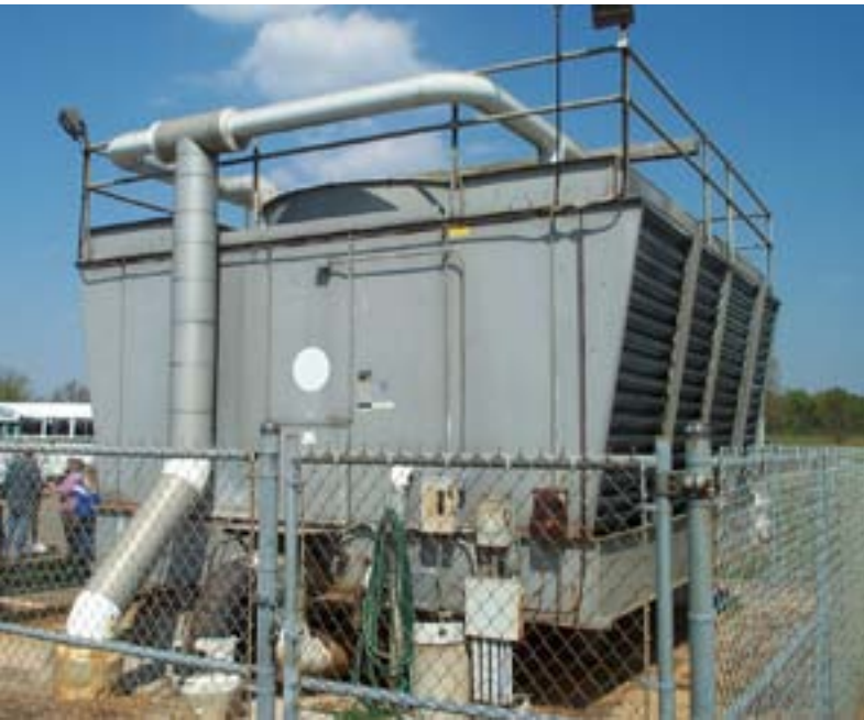
The insulation and windings on cooling tower fan motors must be tested.
