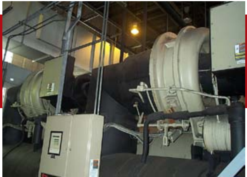
Commonly, a group of centrifugal chillers provides redundancy and step capacity.
