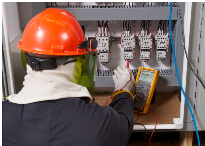
Zach Bryson of Keithly Electric tests for continuity and voltage at the load side of a motor starter overload module using the Fluke 289 True-rms Logging Multimeter.
