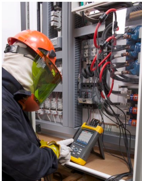
Using the Fluke 435 Three-Phase Power Quality Analyzer, Bryson examines wave forms and harmonics levels on the input side of a motor variable speed drive.
