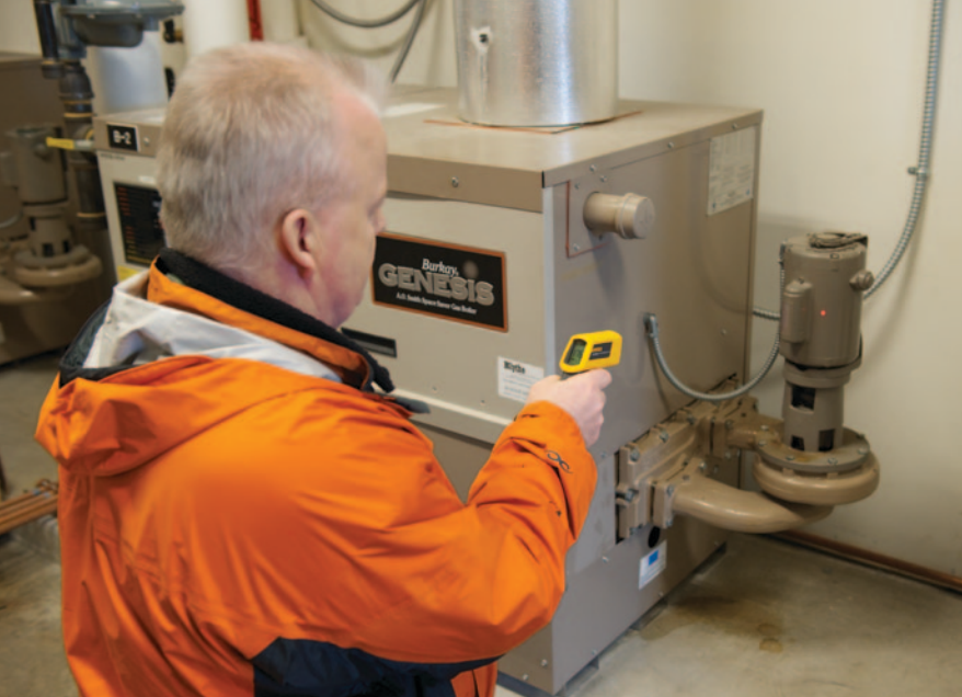
The Fluke 62 Mini Infrared Thermometer helps Anacortes Facilities Manager Russ Pittis search for hot spots that could signal equipment problems.
