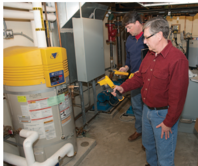
Shared Resource Conservation Manager Ric Boge (foreground) and Paul Tingley, Building and Grounds Supervisor for the City of Burlington, check HVAC facility performance with the Fluke Ti32 Thermal Imager.
