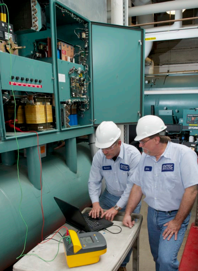
Bernie Kargol (left) and Mike Schum download and discuss data from the Fluke 1555 Insulation Resistance Tester after running tests (when the chiller is powered off) on one of several chillers at a large hospital.
