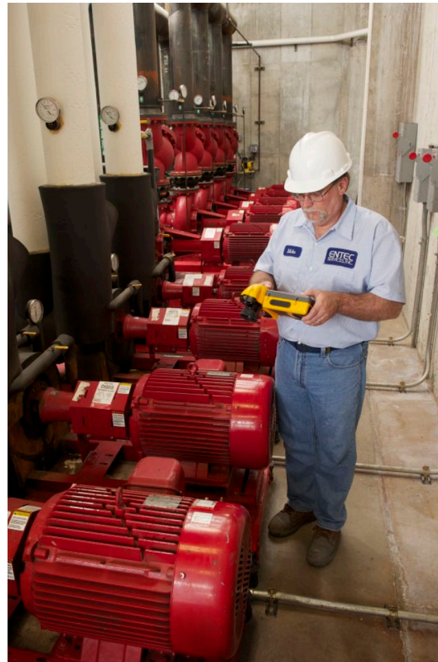
Mike Schum uses a Fluke Ti45FT Thermal Imager to compare performance across an array of motors and pumps. Next to Mike, the chilled water pumps move chilled water to and from the air handling units located throughout the hospital. Behind him, the uninsulated condenser water pipes move condenser water to and from cooling towers.
