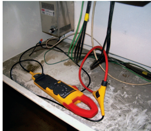
The iFlex™ probe surrounds a single conductor in this drive cabinet for an air handler unit (AHU). The Fluke 381 Clamp Meter is used to record the amperage reading to troubleshoot a suspected drive problem. The same clamp meter is used to estimate the horsepower produced by a motor.
