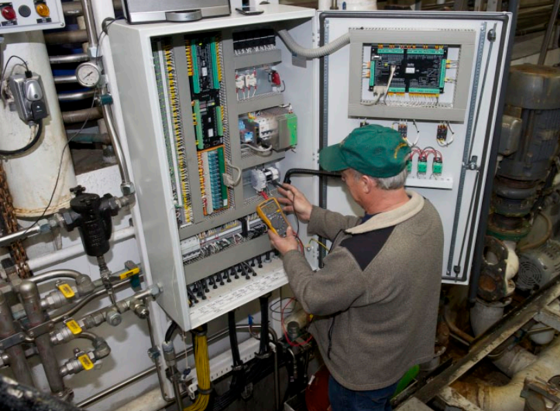
Taking measurements in a programmable logic control (PLC) panel on the Starbound.
