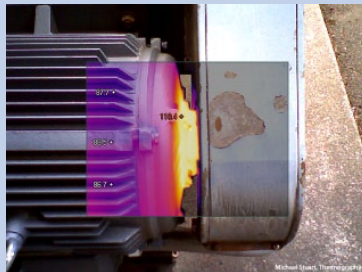
Overheating motor with winding issue.
