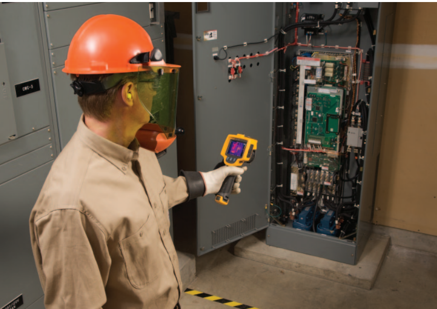
Inspection with the Fluke Ti32 Thermal Imager can reveal defective components and maintenance issues, such as energy-wasting loose connections.
