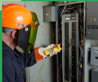
Wood uses his Fluke 337 Clamp Meter to verify that amperage available at the panel is adequate to supply the charging station.
