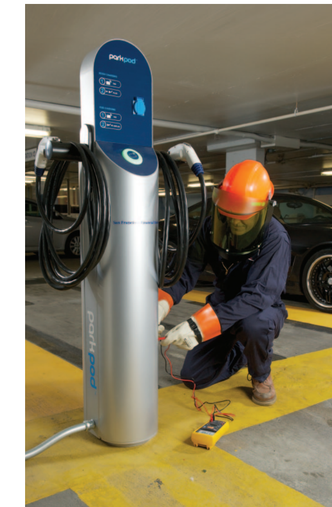
Keith Wood checks the voltage available at the ParkPod charging station, using his Fluke 1587 Insulation Multimeter.
