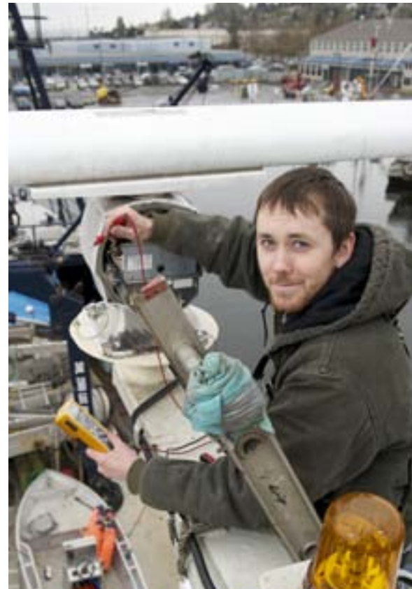
High above the harbor, field electronics technician Jeff McMahon tests power supplied to a radar antenna.
