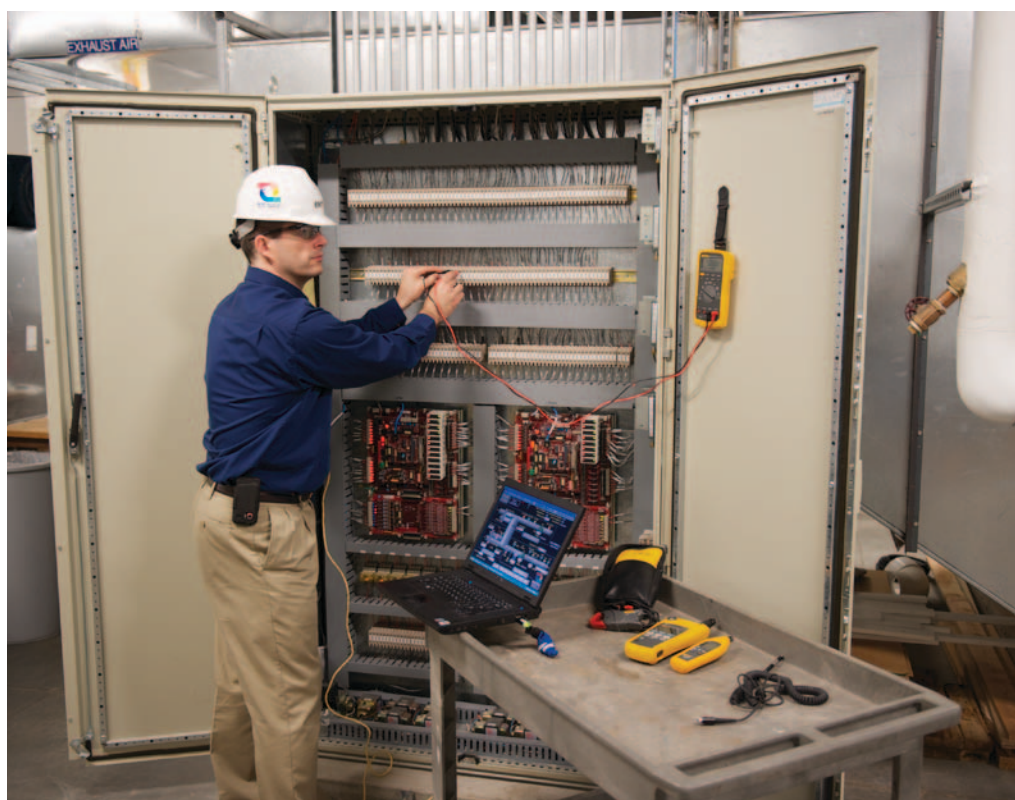
Mark Janco, System Specialist for ENTEC, uses his laptop with the Fluke 87V to tap into the Figge’s building automation system to run routing checks of various low-voltage HVAC system control centers.
