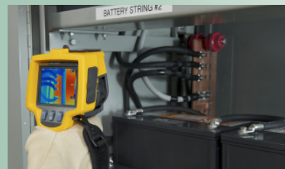
Checking the contact buss in the back of a battery bank cabinet (these lugs are tight). With a thermal imager, hands stay out of the cabinet.
