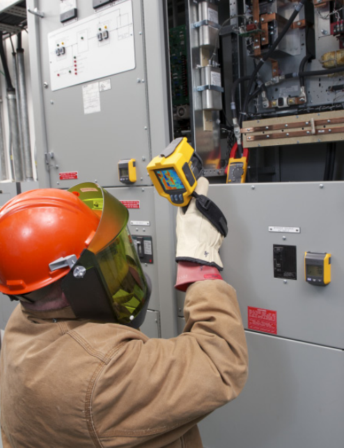
Jerry uses a Fluke Ti32 Thermal Imager to check every component of a UPS system, looking for loose connections, heat dissipation, and overall performance.
