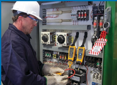
After locking out the main power to the motor control, Chipper Stohl connects his CNX i3000 Current Module and a CNX v3000 AC Wireless Voltage Module in the de-energized cabinet.
