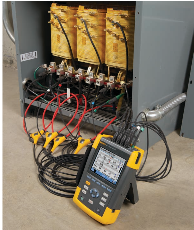
Use a power logger such as this Fluke 434 II Energy Analyzer to measure the fiscal cost of energy wasted due to poor power quality.
