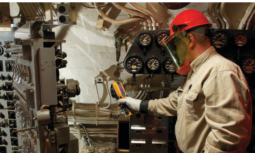
The control room is the center of the submarine, both physically and operationally. Bill uses a Fluke Ti125 to look behind the IC switchboard, which has both 120 volt ac and 120 volt dc systems.
