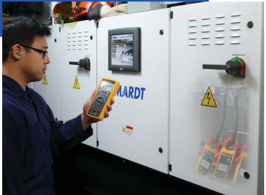
Using the Fluke CNX™ 3000 wireless system to take a three-phase live electrical measurement, communicating the measurement through the closed panel door.
