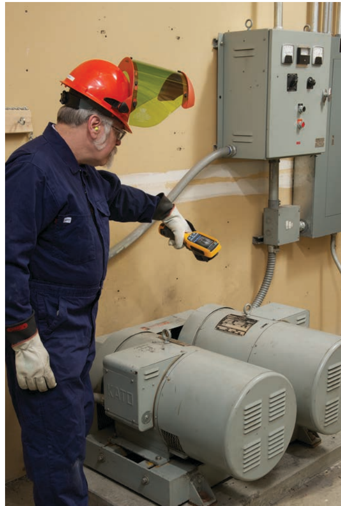
Thermal inspection of electrical and mechanical motor components with the Fluke Ti125 Thermal Imager.
