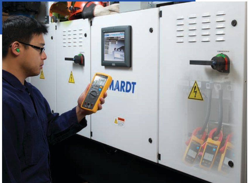
Using the Fluke CNX™ 3000 wireless system to take a three-phase live electrical measurement, communicating the measurement through the closed panel door.
