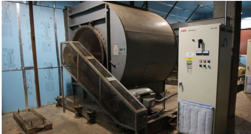
Over time, HVAC systems can become inefficient. Energy logging at the highest loads can help identify wasted energy and potential savings.
