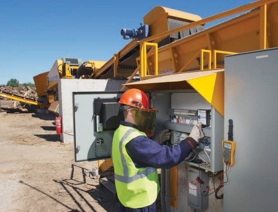
A CBI technician double-checks with his Fluke 117 Digital Multimeter to ensure the proper signals are reading correctly as he commissions a new system.
