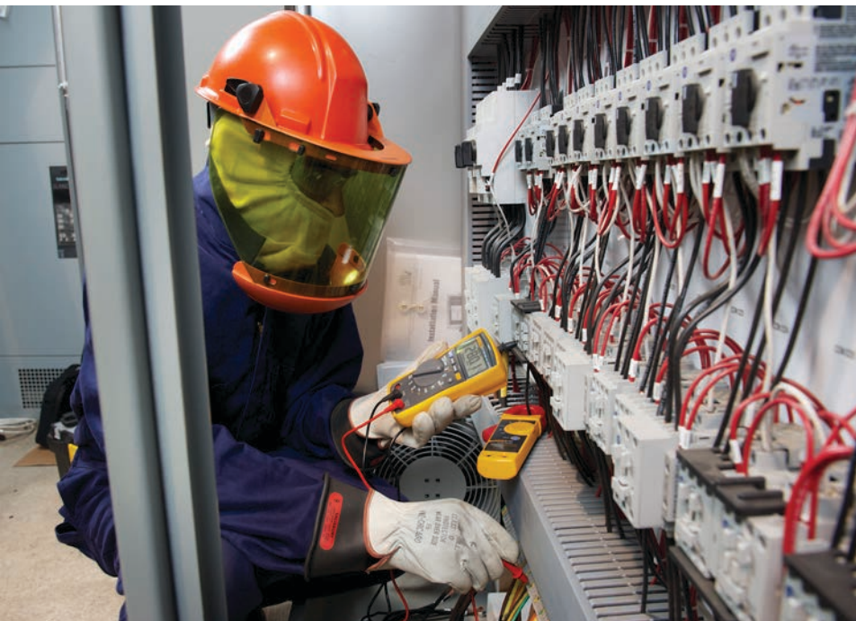
The motor control center is the backbone of the grinding system. Nothing happens at the grinder, 150 feet (45.7 meters) away, unless the power is balanced and running as designed. Although these systems are almost bulletproof, fine-tuning is needed as the CBI technician goes through the commissioning of any new system. He dons his personal protective gear and uses his Fluke 117 Electrician's Digital Multimeter and Fluke 322 Digital AC Clamp Meter to take measurements.
