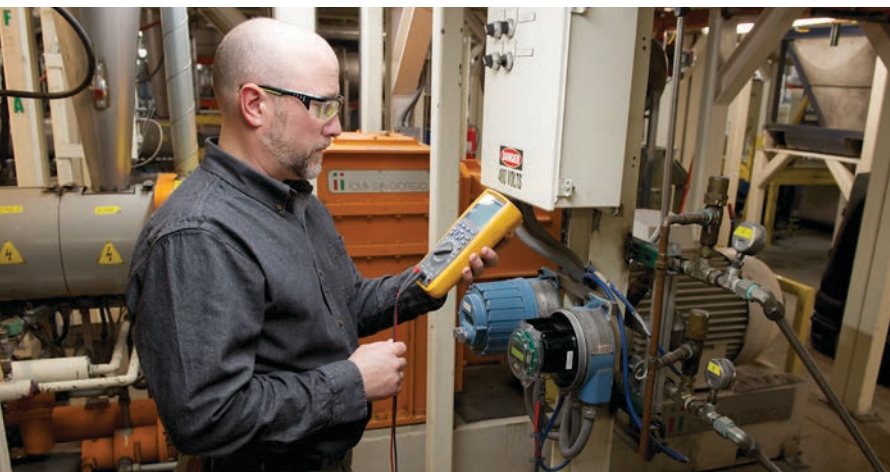
The Fluke 289 has the accuracy Derek needs to troubleshoot the 24 volt signal inside this flow transmitter intrinsically safe enclosure, which controls the flow rate of an extrusion machine.
