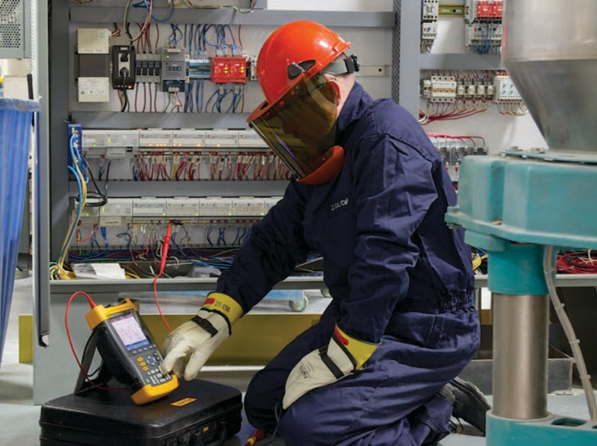
The Fluke 199C ScopeMeter is Derek Forsythe's tool of choice when he needs to check the signal response on this material feed control panel. Derek always makes the choice to work safe. Even though this cabinet is rated at a category 0 arc flash hazard, Derek suits up and uses proper PPE, just in case.
