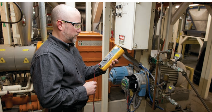
The Fluke 289 has the accuracy Derek needs to troubleshoot the 24 volt signal inside this flow transmitter intrinsically safe enclosure, which controls the flow rate of an extrusion machine.
