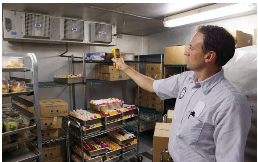
Mark uses his 62 MAX Infrared Thermometer to check refrigeration units in a walk-in cooler, as part of his preventive maintenance program.
