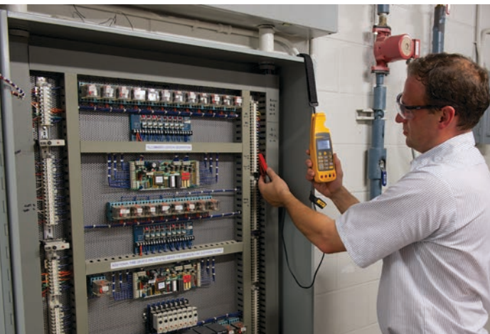
With his Fluke 773 Milliamp Process Meter, Mark checks the control signal loop in the low-voltage relay cabinet.
