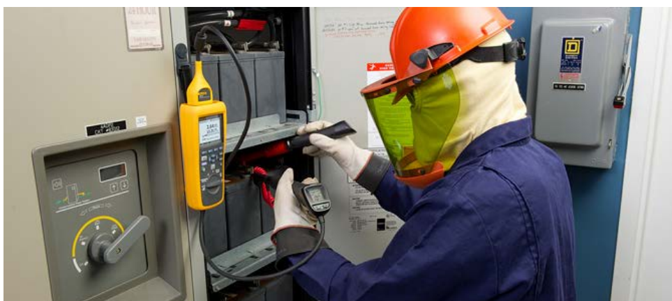
Using the Fluke BT52X to measure impedance, for the quarterly cell/unit internal ohmic value test.
